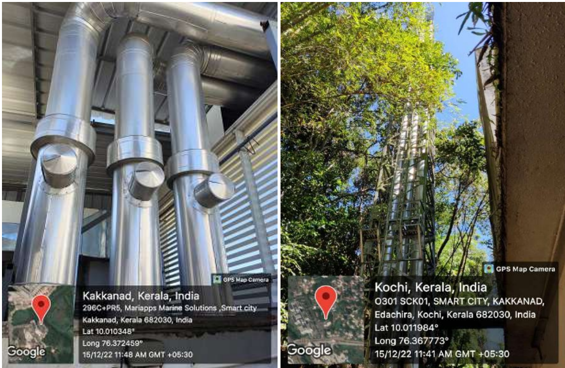
Stack of DG
