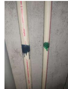
Dual Plumbing Lines
